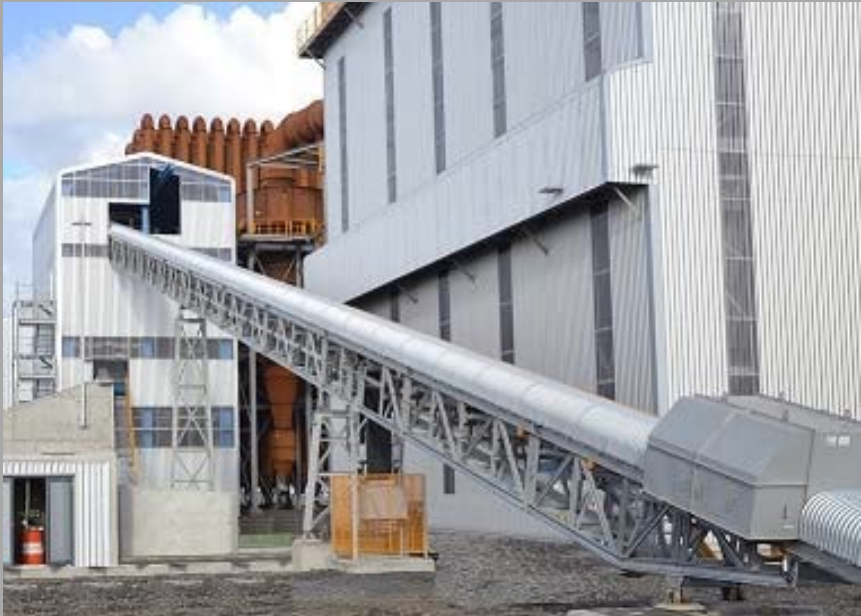
DOSING BELT CONVEYOR FOR MATERIAL EXTRACTION
